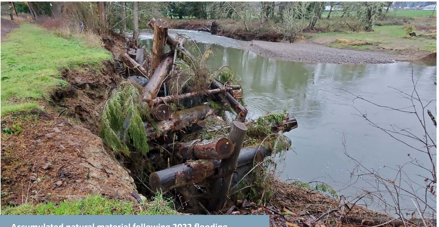
Accumulated natural material following 2022 flooding.
